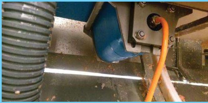
Centre drive arrangement multiple pulleys
