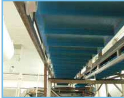
UHMW support on return
