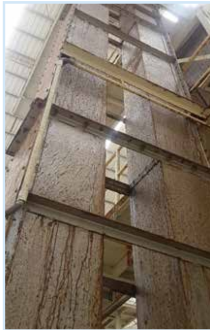
Closed system - cannot be cleaned
